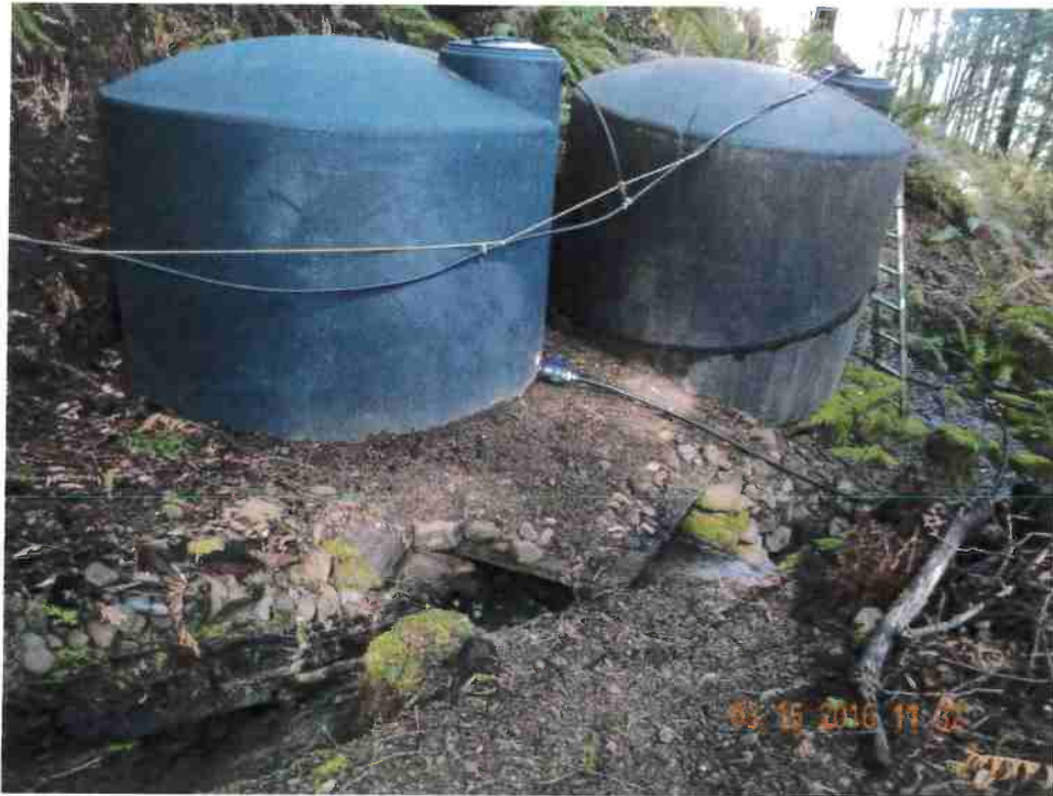
Figure 4. Two 3000-gallon storage tanks located at POD.
