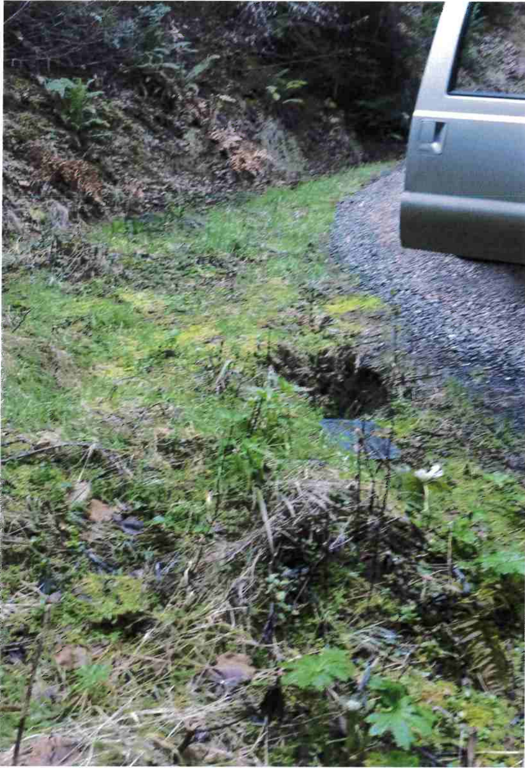
Figure 8. Inlet at 12" pipe at STX-1. Culvert will be replaced with a 24" diameter pipe.
