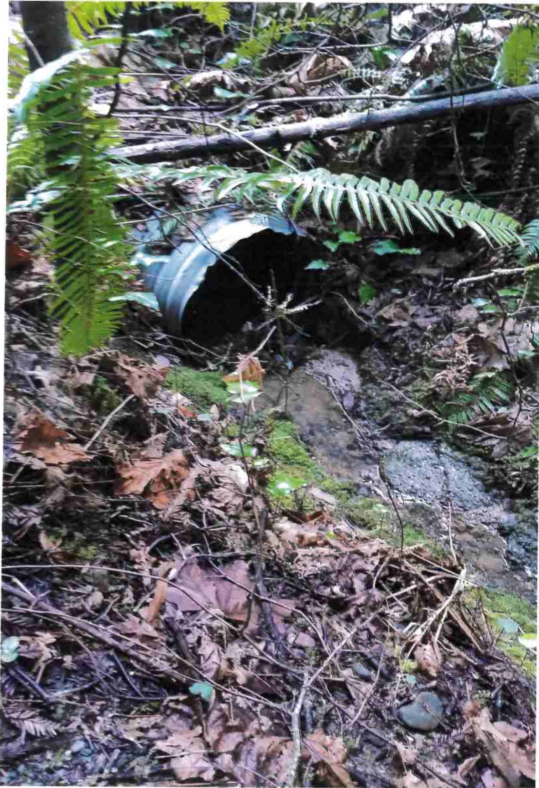
Figure 10. Inlet at 18" CMP at STX-2. Culvert will be replaced with a 24" diameter pipe.
