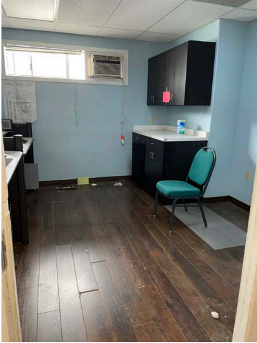
Existing floor in former dispatch office. Flooring failing at most joints.
