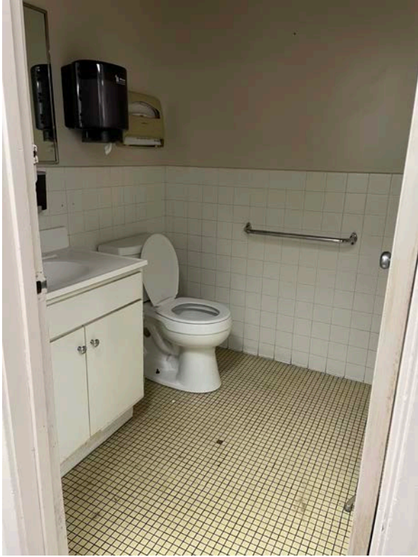
Existing bathroom showing cracked tile flooring. Failing lights and ceiling fan not shown.
