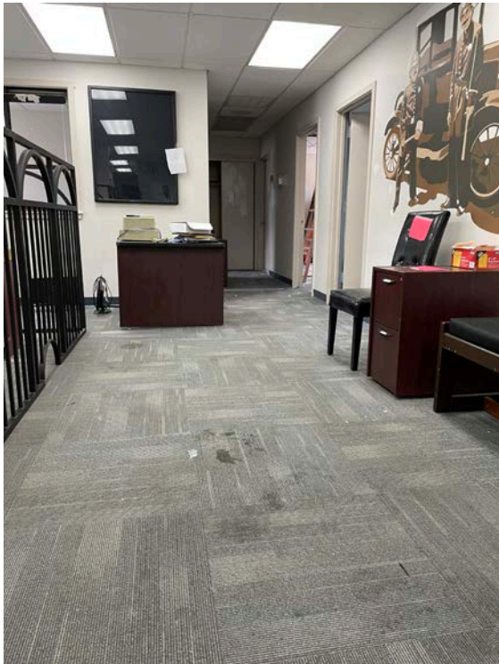
Existing reception area carpet showing wear and staining.
