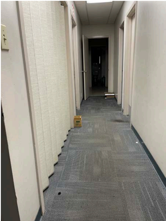
Existing hallway showing carpet wear and staining.
