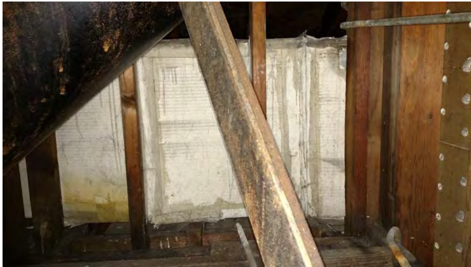
TSI Air-Cell Wrap On HVAC Duct In Attic
