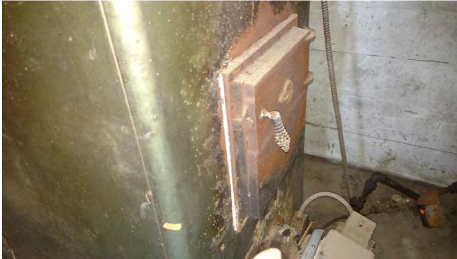
TSI Gasket On Door Of Boiler In Boiler Room
