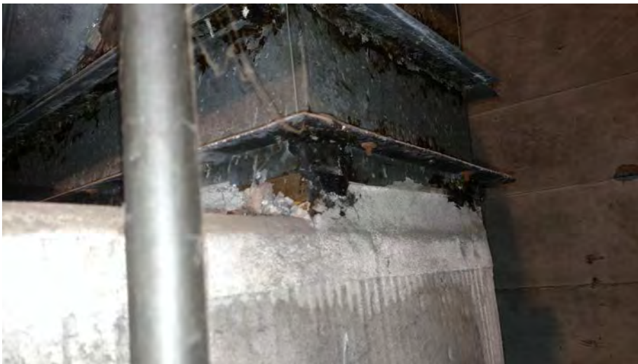
TSI Air-Cell Wrap & Black Caulking On HVAC Furnace/Duct In Boiler Rm
