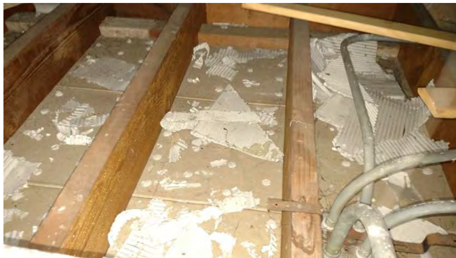
TSI Air-Cell Wrap Debris On Ceiling In Attic
