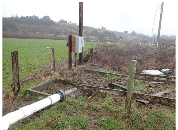
View of electrical box for the water pump
