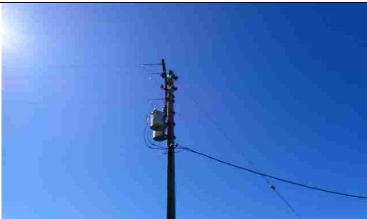
View of the pole mounted transformer
