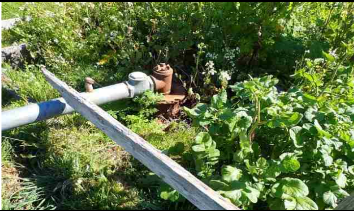
View of the water pump
