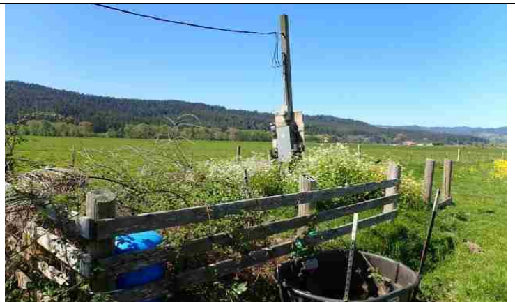
View of electrical box for the water pump
