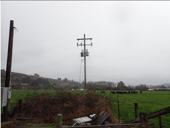
View of the pole mounted transformer
