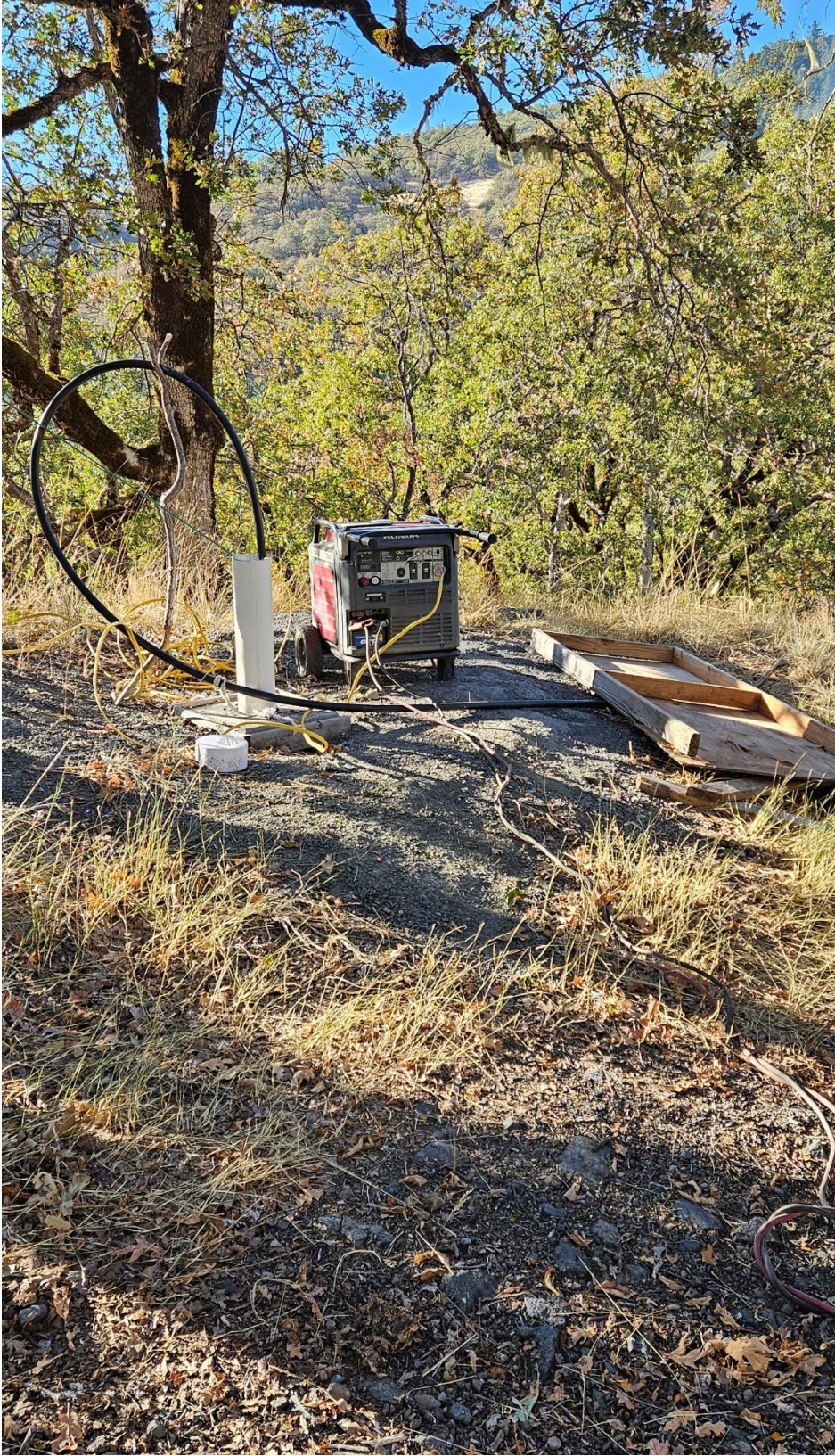
Well/Generator on parcel 208-241-011-000
