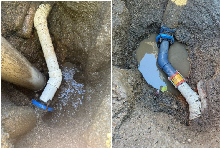
Photo Inset Below: Leak on East College Ave
