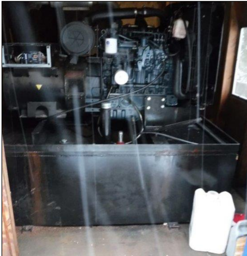
Photo 3. Diesel generator with shed and containment.
