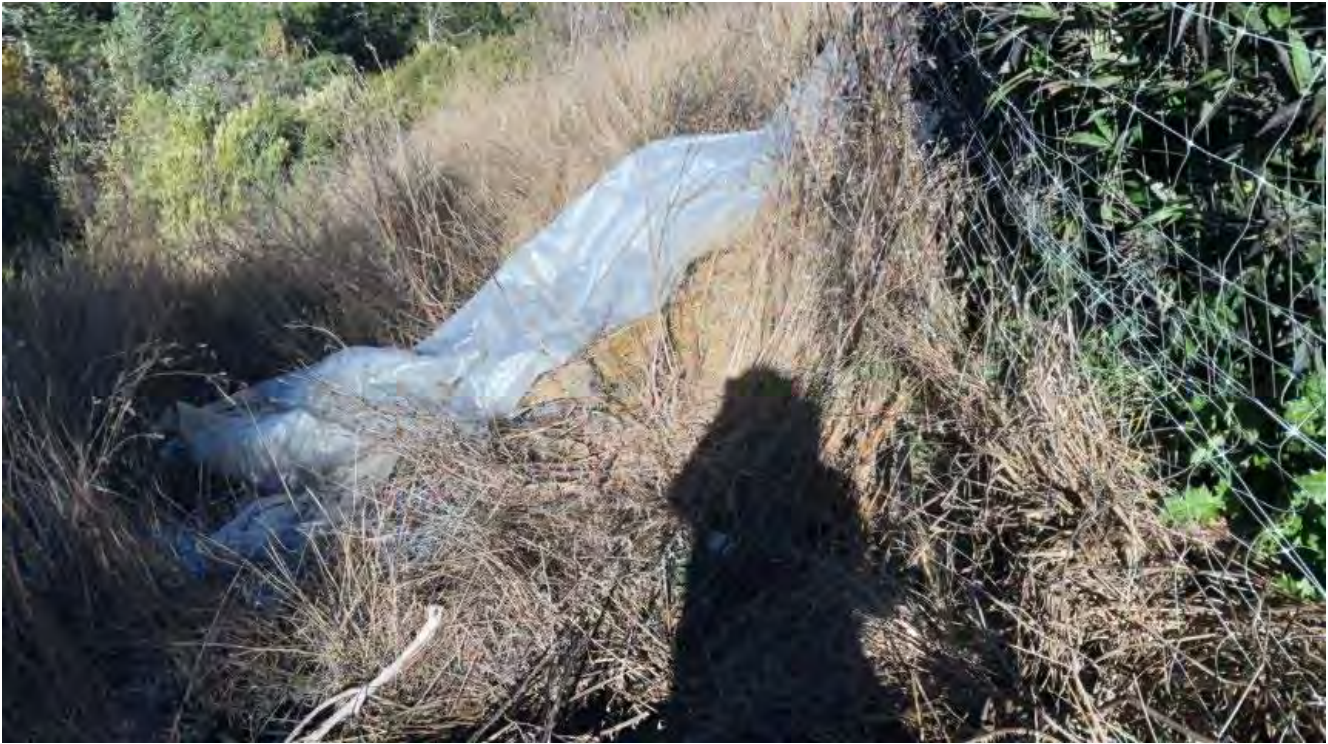
Fig. 7.1 Fill slope of CA2 with two foot vertical displacement of the fill. Violation/Remediation point not specified by NCRWQCB, labeled Fig 20. Photo by NCRWQCB, 24 October 2024.
