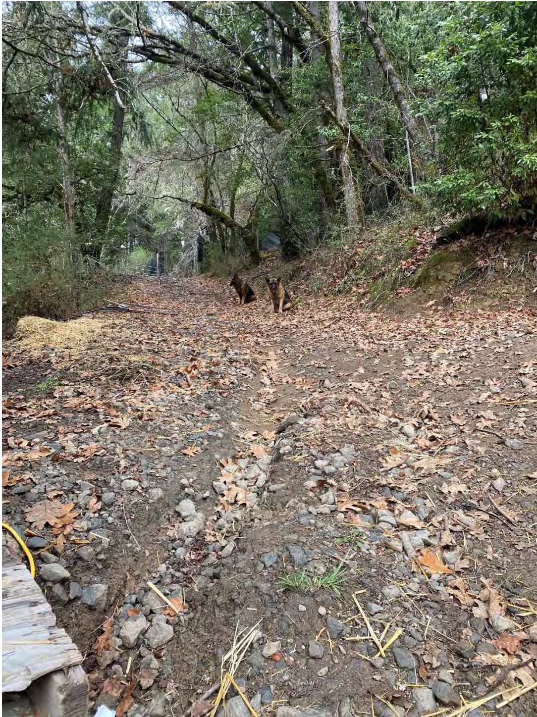
Fig. 4.5 Drainage improvements draw storm water away from CA2. Photo by Permittee, 20 December 2024.
