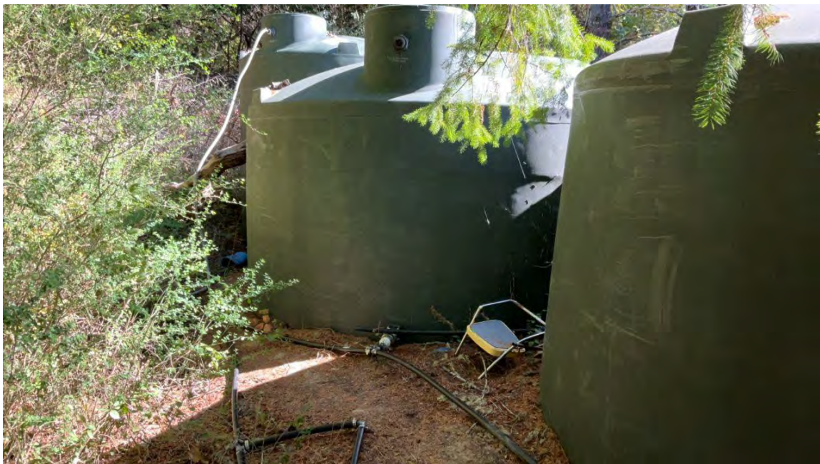
Fig. 16.2 The surface water diversion line from Point 2 connects to water storage tanks above CAI at Point 16 and appears to be used to irrigate. Photo by NCRWQCB, 24 October 2024.
