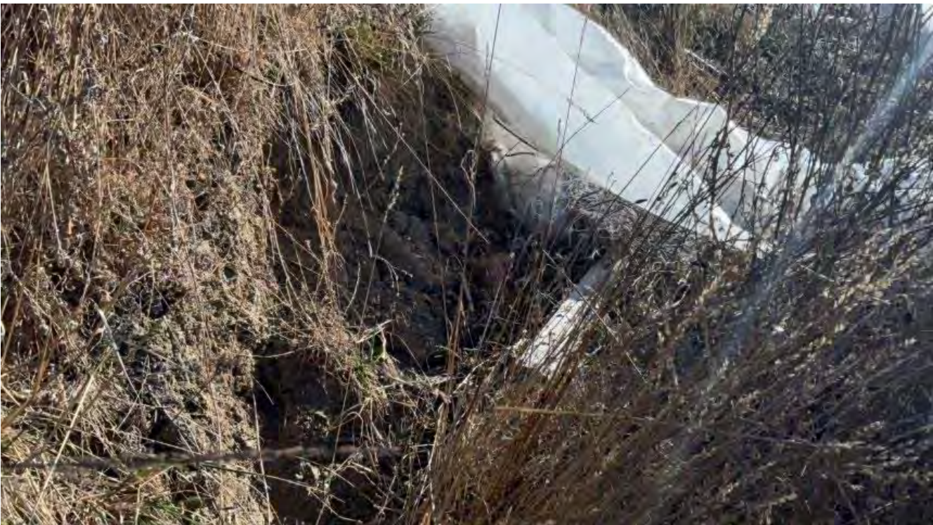
Fig. 7.2 CA2 with two vertical displacement of the fill. Violation/Remediation point not specified by NCRWQCB, labeled Fig 21. Photo by NCRWQCB, 24 October 2024.
