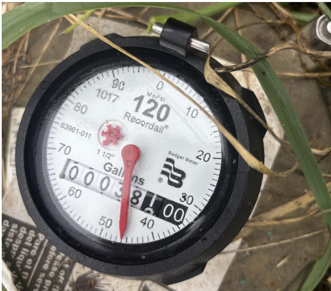
Figure 1: Water meter on permitted well diversion clearly indicating 38,146 gallons. Model 120 measures 100,000,000 gallons.
