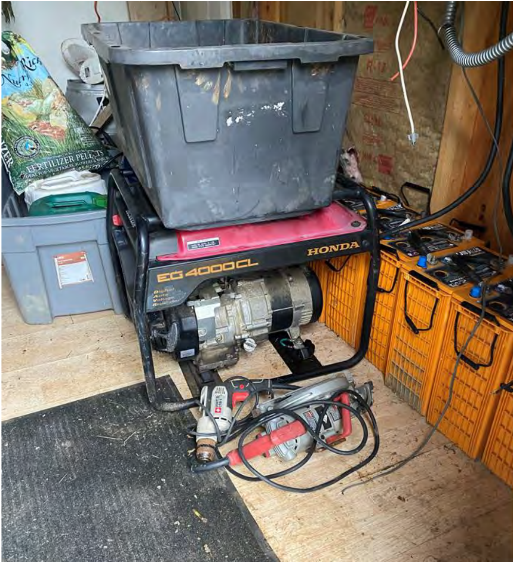
Fig. 14.2 Generator stored indoors when not in use. County officials recommended kiddie pool as secondary containment when in use outside. Photo by Permittee, 20 December 2024.
