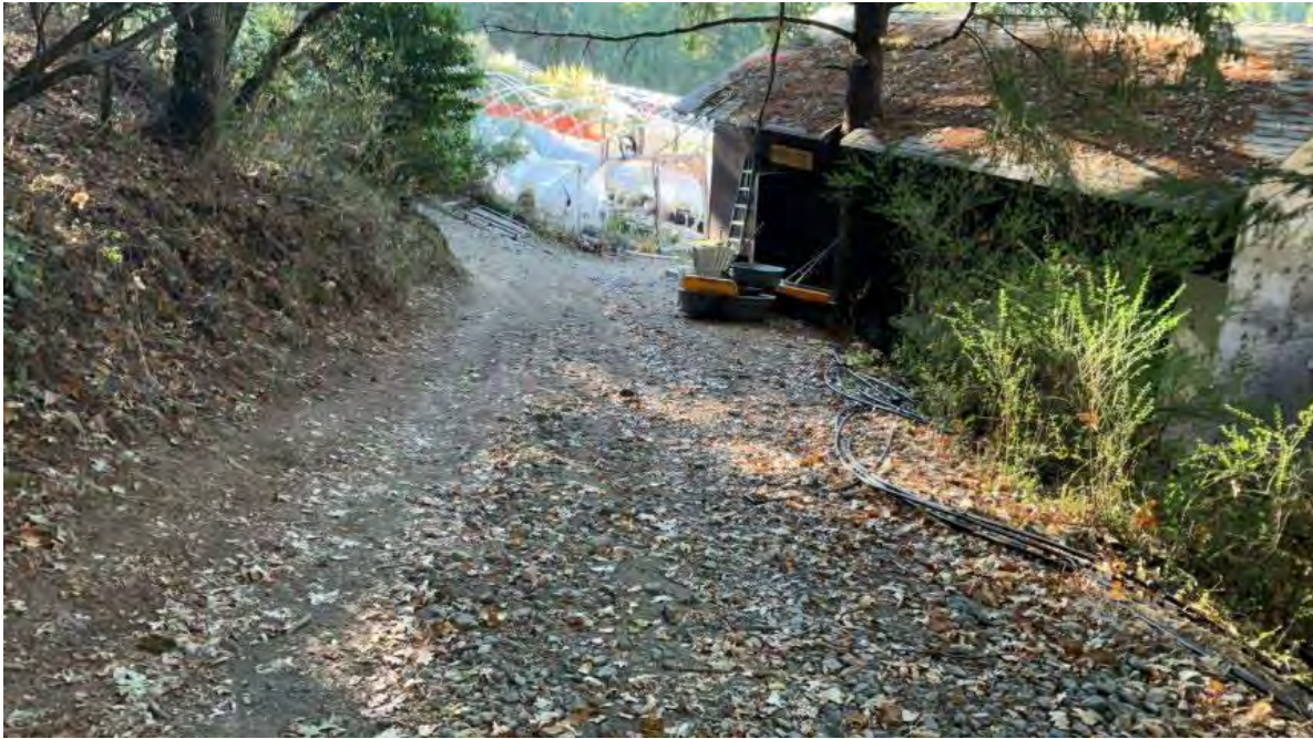
Fig. 4.1 Driveway to CA2 is steep and lacks drainage; stormwater runoff is concentrated into the cultivation and storage area. Photo by NCRWQCB, 24 October 2024.
