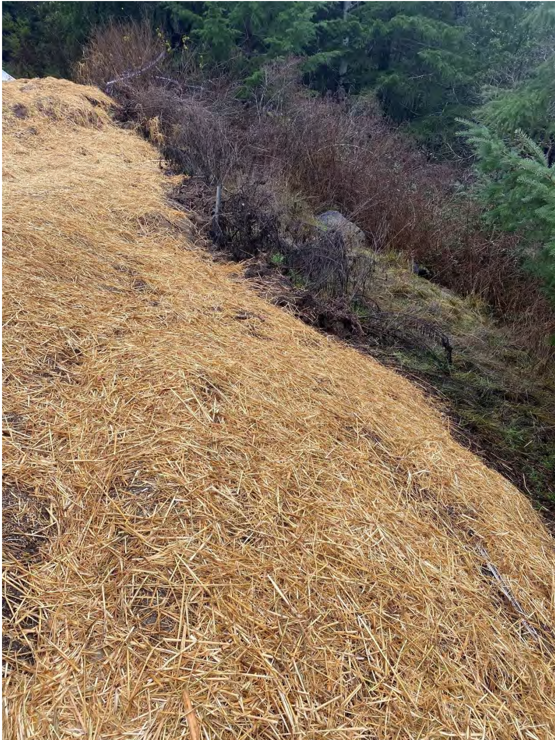
Fig. 7.4 Erosion control implemented at fill slope near CA2. Photo by Permittee, 20 December 2024.
