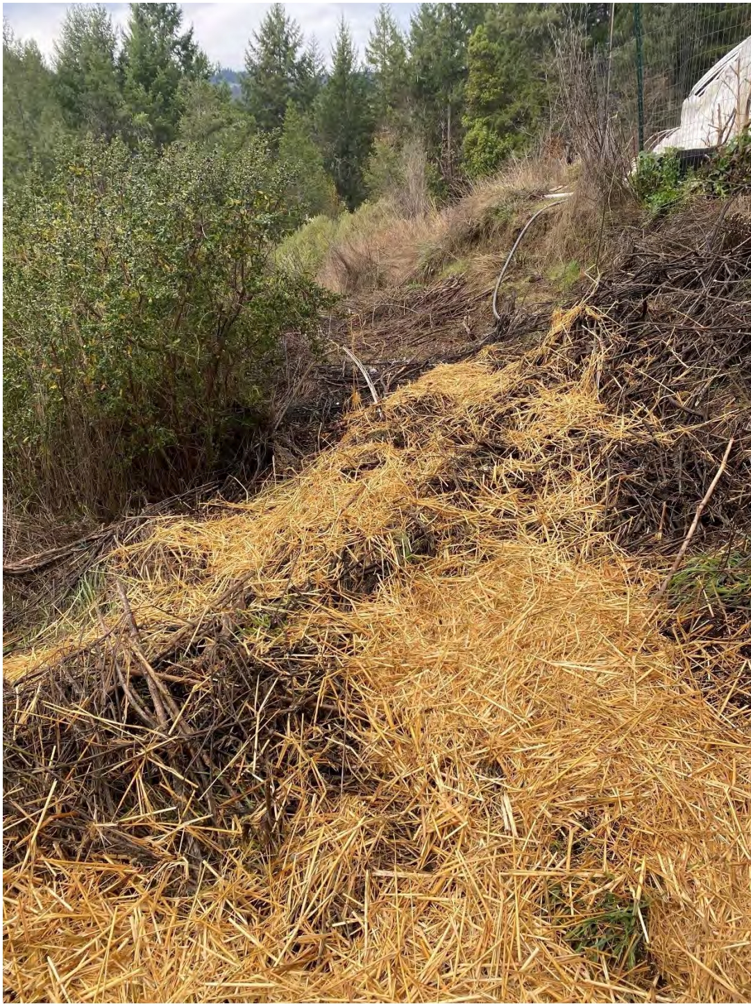
Fig. 7.3 Erosion control implemented at fill slope near CA2. Photo by Permittee, 20 December 2024.
