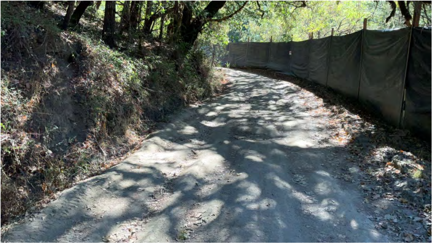
Fig. 12.4 The access road ditch and rilled road surface poses threat of sediment delivery to the stream crossing at Point 12. Photo by NCRWQCB, 24 October 2024.
