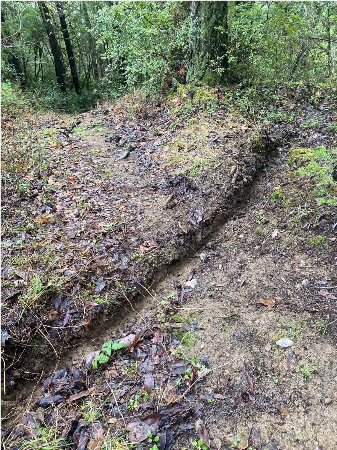
Fig. 3.2 Water bar recut. Photo by Permittee, 20 December 2024.
