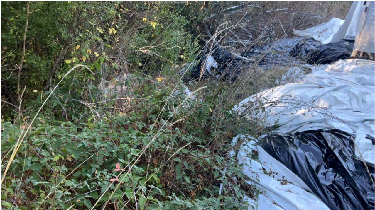
Fig. 8.2 Refuse from CA2 is accumulated at the edge of the 50 foot setback to the Class III watercourse. Violation/Remediation point not specified by NCRWQCB, labeled Fig 23. Photo by NCRWQCB, 24 October 2024.
