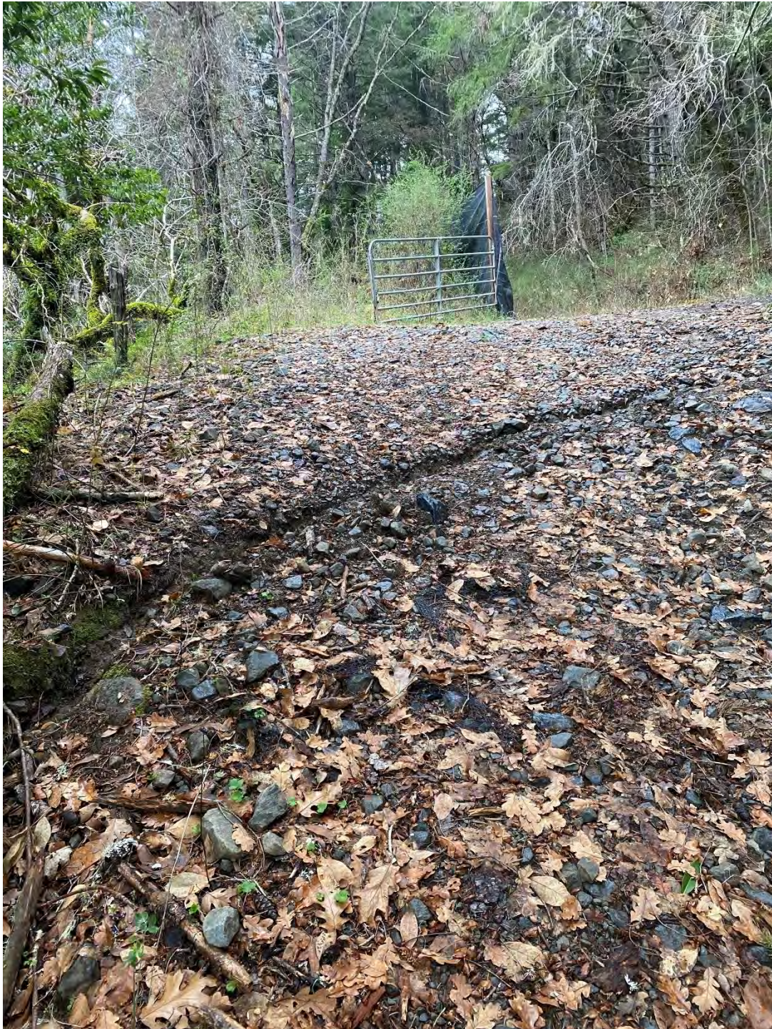
Fig. 4.4 Drainage improvements draw storm water away from CA2. Photo by Permittee, 20 December 2024.
