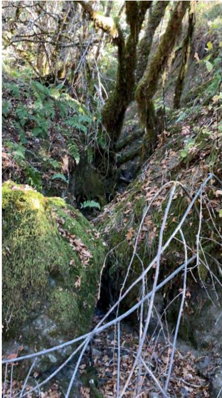
Fig. 12.1 Class III watercourse upstream of road crossing at Point 12. Photo by NCRWQCB, 24 October 2024.
