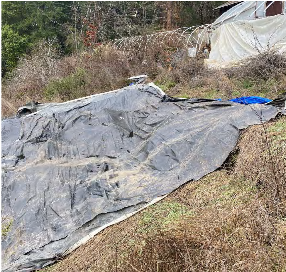
Fig. 5.4 Potting soil covered on fill slope of the graded flat at CA2. Photo by Permittee, 20 December 2024.
