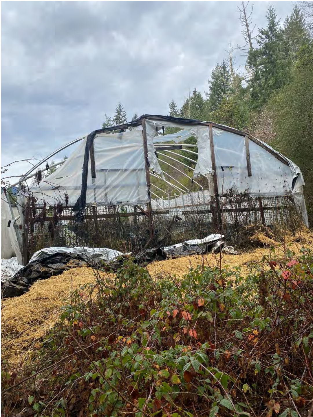
Fig. 8.7 Refuse mitigation performed by Permittee; dump receipts attached. Photo by Permittee, 20 December 2024.
