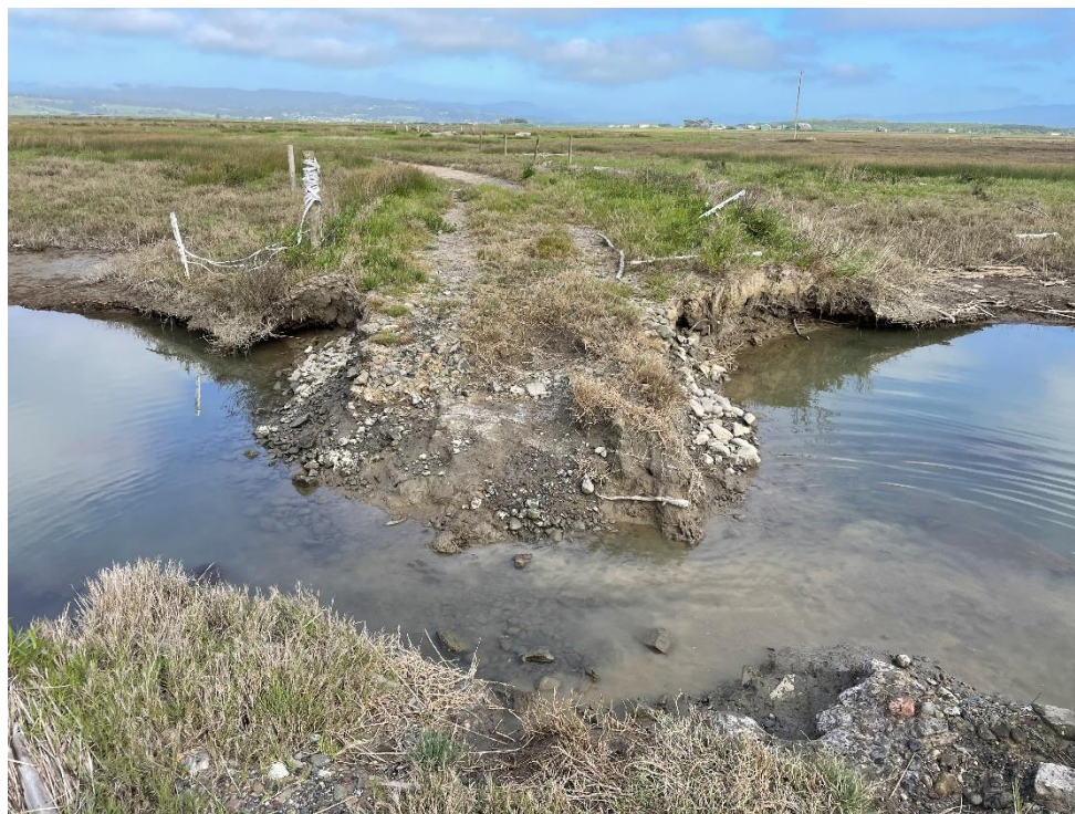
Photo 8—View of failed road crossing on Senestraro Lane (looking northeast) and the large interior slough (unnamed) that now passes over it.
