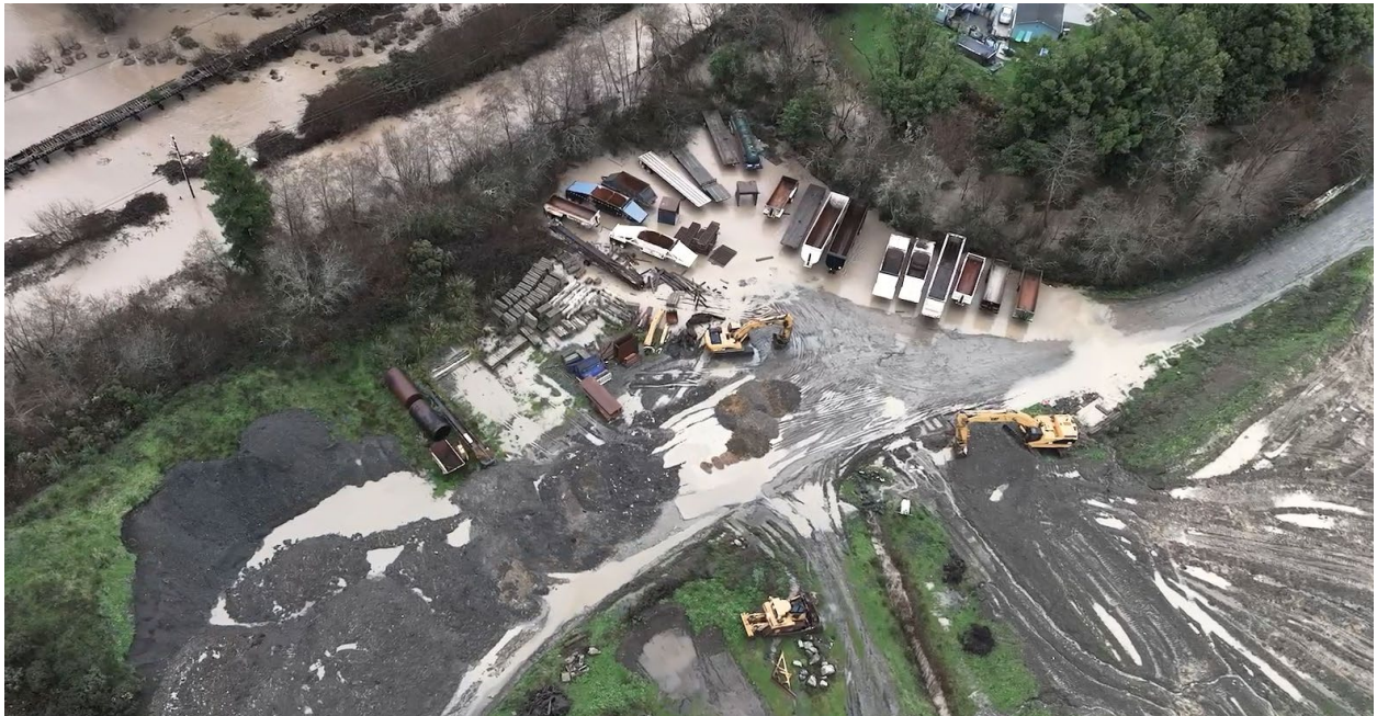
The area where the new, unpermitted berm has been constructed.
