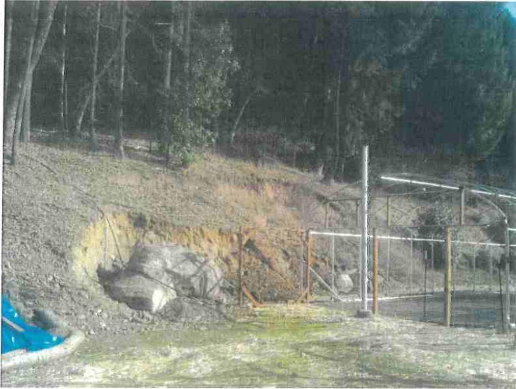
Figure 3 Stabilization of Upper Cut Bank Failure
