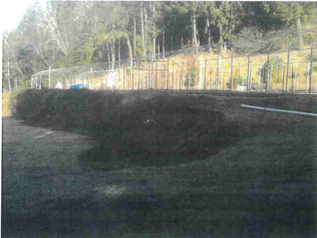
Figure 4 Lower Terrace Cut Bank Failure
