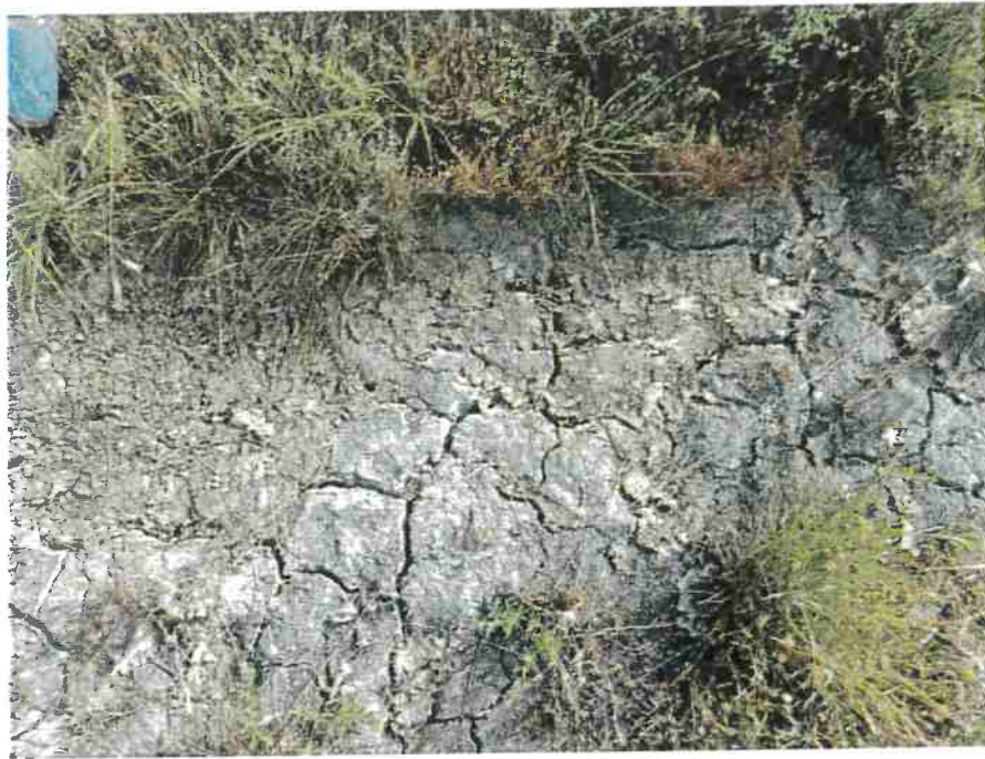
Figure 3: Surface cracks at W-1 taken on 7/9/19.
