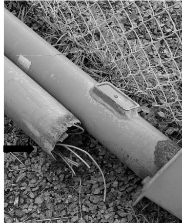
Image 2: Fallen rusted and corroded light pole.
