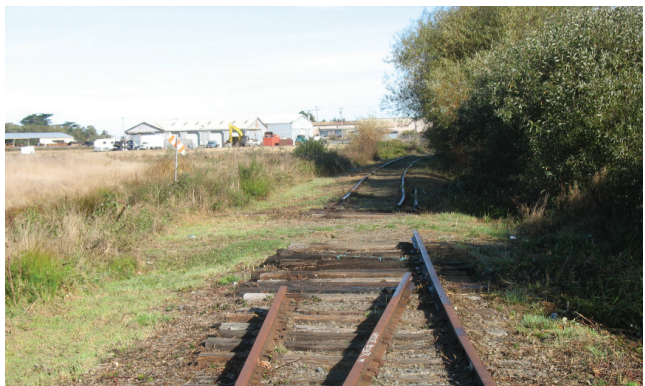
View of missing tracks in rail corridor looking north
