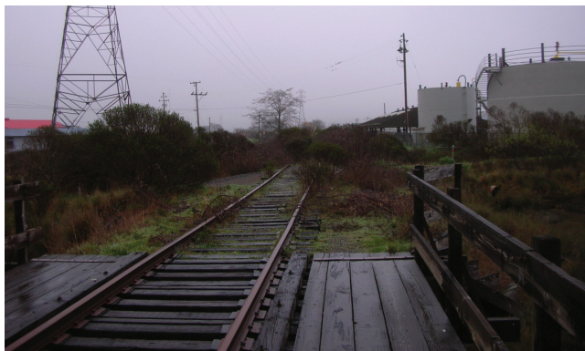
Looking southeast towards City Corporate yard from bridge at Jolly Giant Creek
