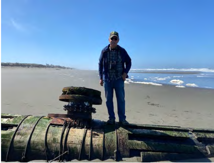
Image 3: Degraded outfall pipe showing...
