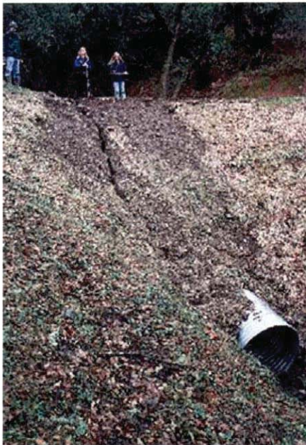
Figure 41. Fill surface erosion occurring after a road upgrading project. Photo: Bill Weaver, Pacific Watershed Associates.
