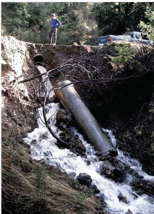
Figure 34. Outlet of a concrete culvert (30 inches in diameter) before the project. The culvert was placed too high in the fill, resulting in a 10-foot drop to the channel at the outlet. This caused erosion of the road fill and stream banks, eventually undermining the outer section of the culvert. Photo: Jared Gerstein.
